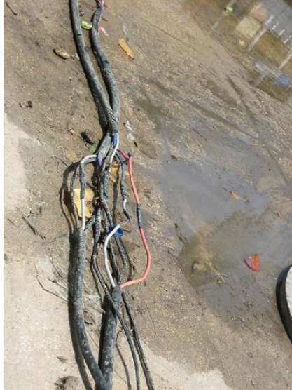
Figure 4: Frayed wires and power cables pose a significant electrical hazard. Image courtesy of marblegravy, Flickr.
