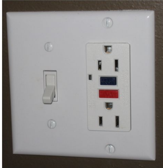
Figure 6: Example of ground fault circuit interrupter. Image courtesy of University of Saskatchewan.
